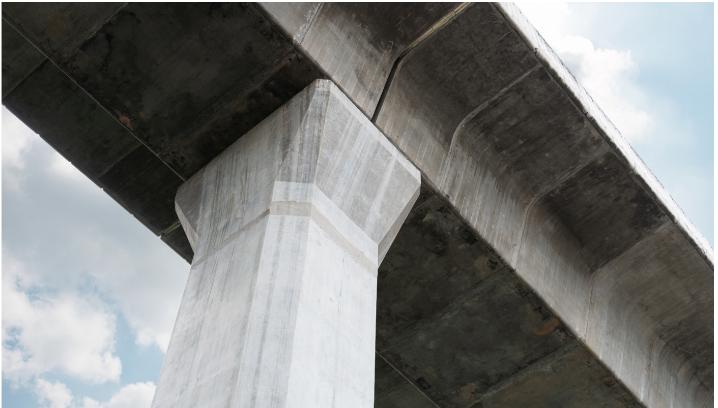
Concrete elements infrastructure
